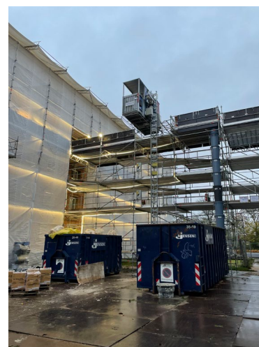
Figure 2: Façade scaffolding and platform between Buildings
