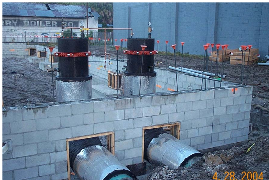
Figure 2. Step downs in the wall footer allowed for proper utilities crossing – Team decision
